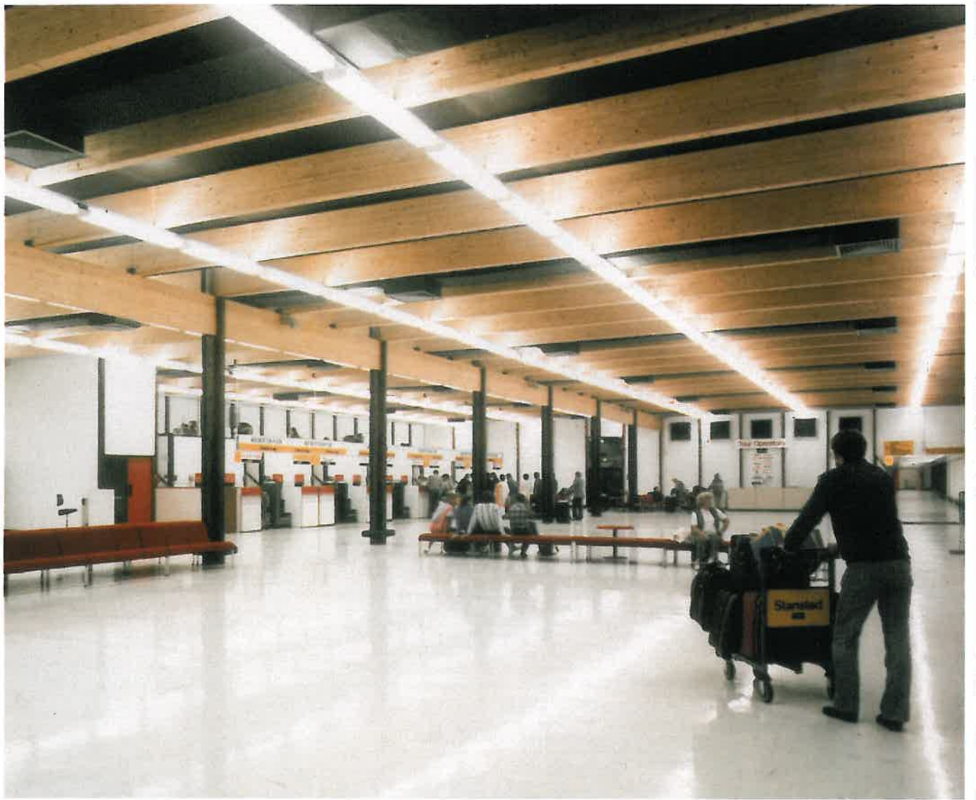
One hundred and eighty twin 1500mm fluorescent luminaires, with electronic ballasts, light the BAA's new terminal building at Stansted Airport. The electrical load, so vital with 24 hour operation, is a mere 20kW and service illuminance 600 lux.
